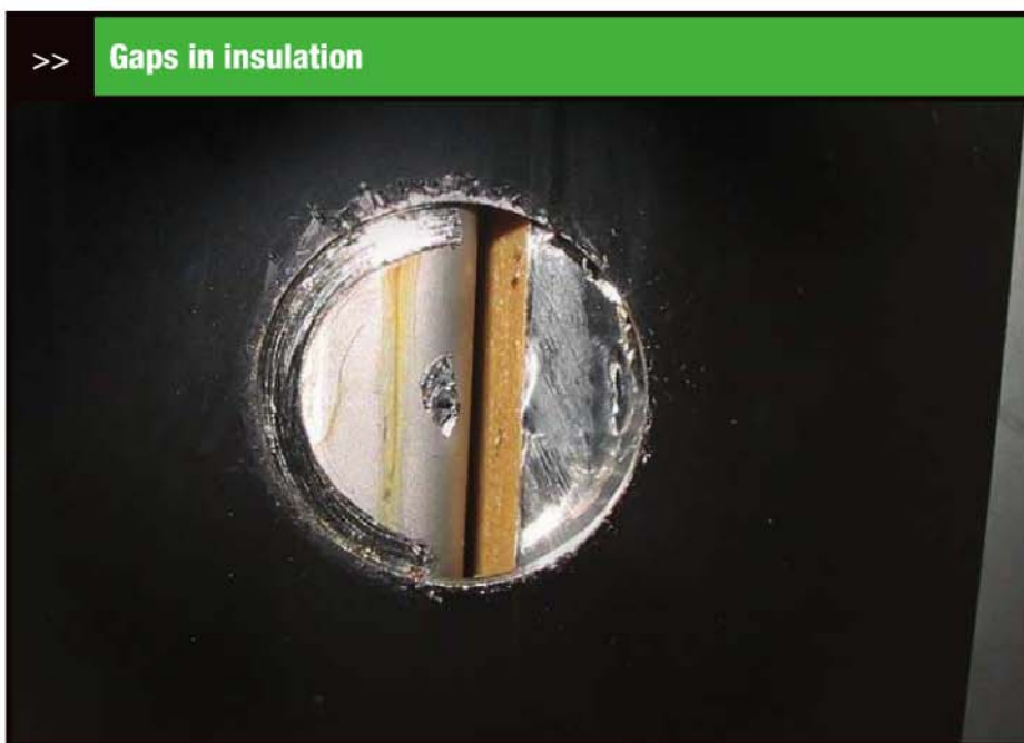
Figure 4. Imaging pinpointed voids in insulation hard to precisely locate otherwise.
