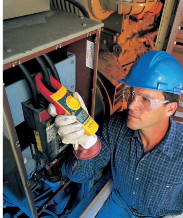
Figure 7: Measuring the loads on a power disconnect.
