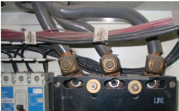
Figure 5: 3-phase power disconnect.
